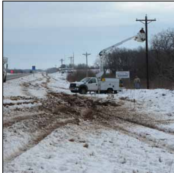
Restoration efforts were hindered by the muddy conditions in Bluestem's service area.
