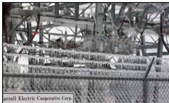
Ice coats one of Carroll Electric's substations.
