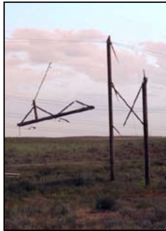
A transmission structure snapped under the force of the wind storm.
