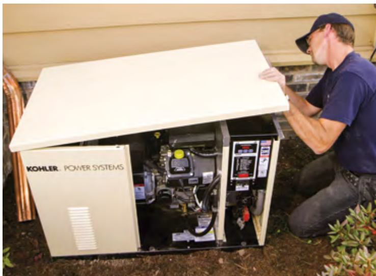
This is a whole-house sized standby generator being installed at a home. Notice the small gas engine inside the housing.
